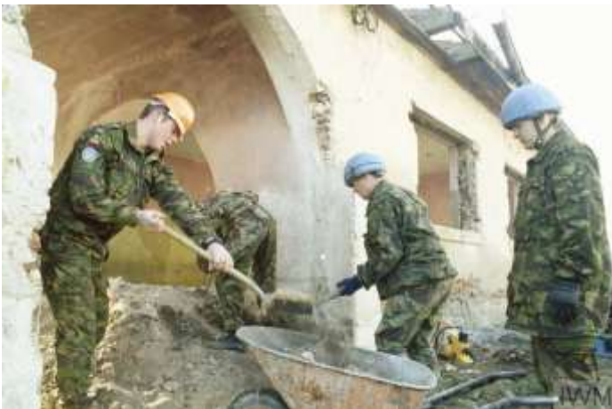
Stari Bila School near Vitez, one of many schools destroyed during the war. (In this photo, members of the Royal Engineers are helping rebuild it.) ( https://historycollection.com/the-brutality-of-the-bosnian-war-reflected-in-these-heartbreaking-photographs/2/ )
